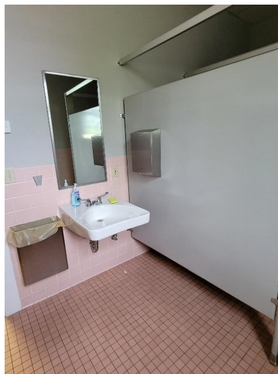
Handicap Accessible Sink
