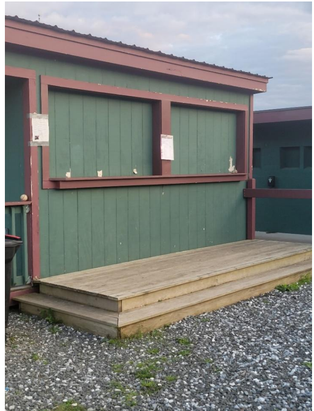
Concession Stand – no accessible route
