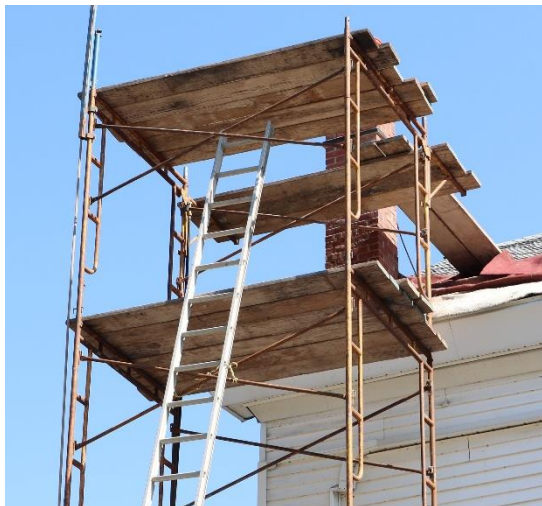
Chimney repairs are a common use of Community Development Block Grant funds.
