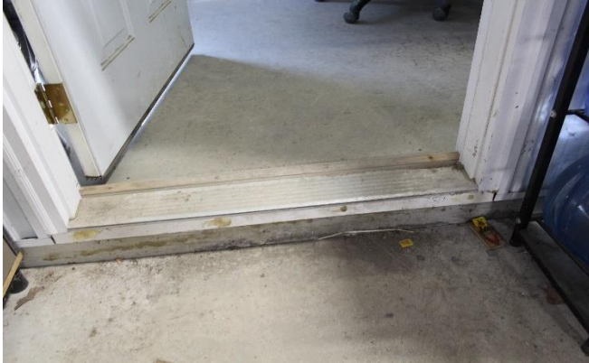
There are obstructions in each passageway from garage to garage.
