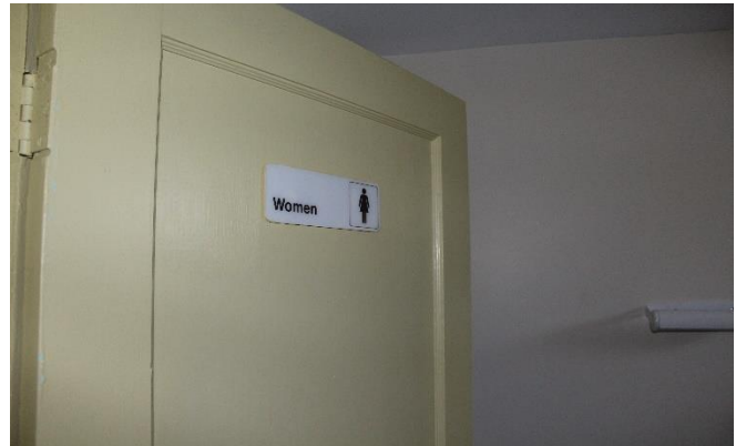
The signs are not tactile and are placed too high above the ground.
