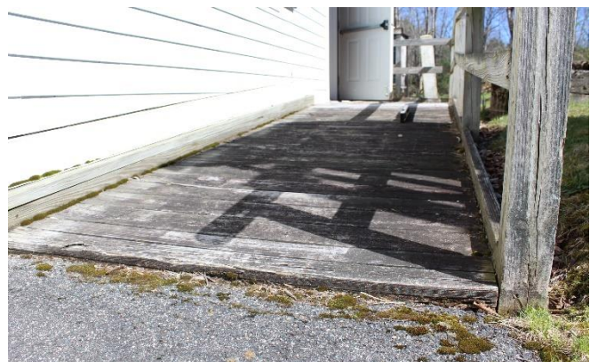
The wooden ramp for handicapped access is out of compliance with the 2010 ADA Standards.
