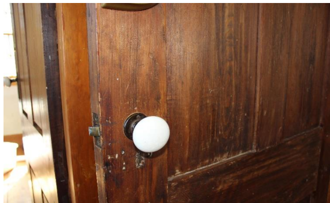
All the upstairs doors have doorknobs, which are not compliant.
