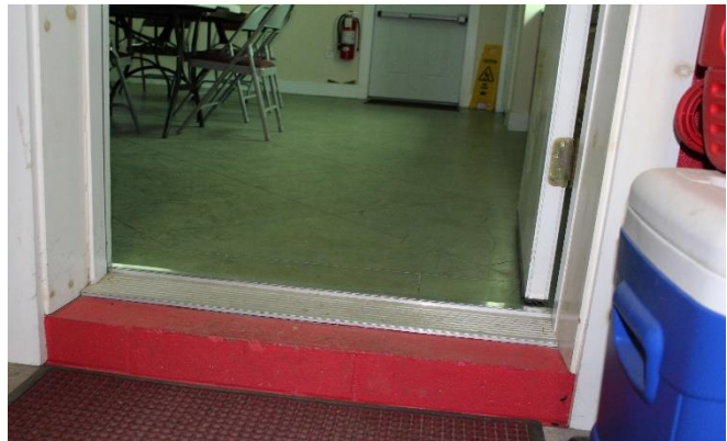
The doorway from the main area to the lounge area requires a significant step up.
