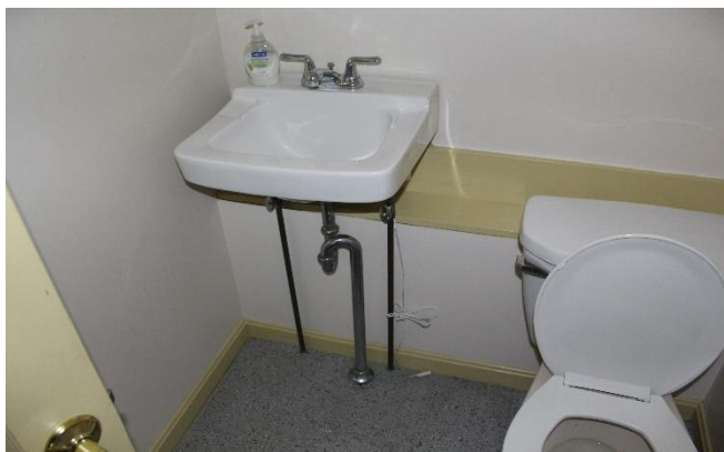
The pipes are exposed in the men’s room. The pipes are covered in the women’s room but there is not sufficient knee clearance.
