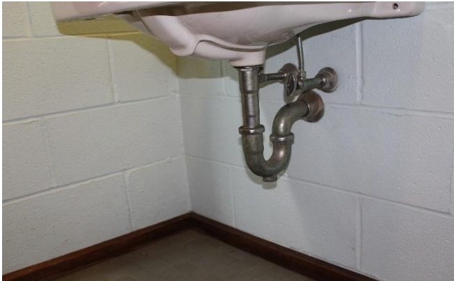
The bathrooms have exposed pipes, which is out of compliance.
