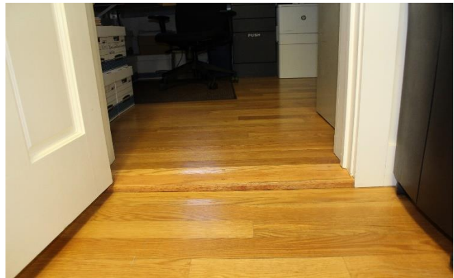
The transition into the Town Clerk’s Office is out of compliance.
