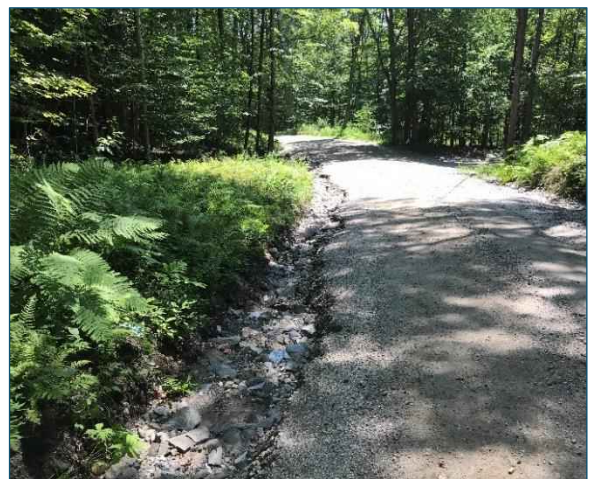
A gully has formed on this steep road because it lacks a constructed ditch or had an insufficiently sized ditch.
