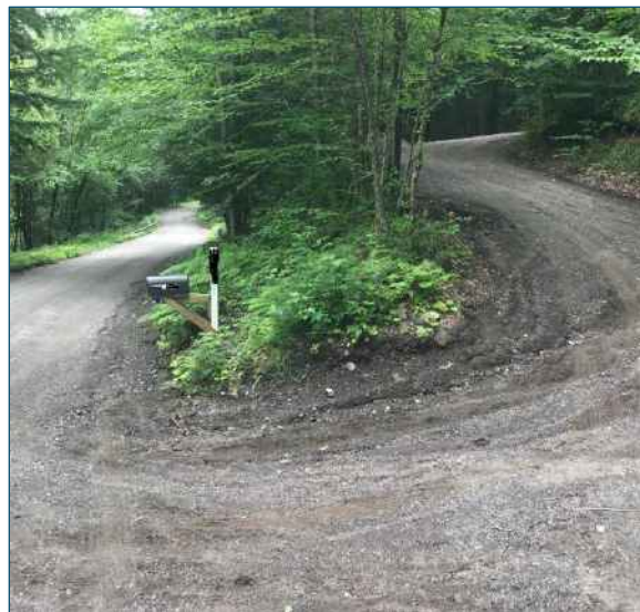
This private driveway is impacting the road by sending runoff to the road and causing the formation of a false ditch.
