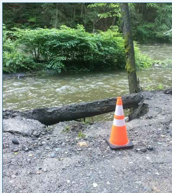
A road shoulder collapsed into a river.
