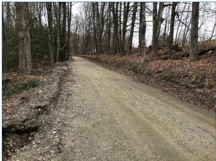
This road is entrenched, and water is eroding off the road in the foreground left.
