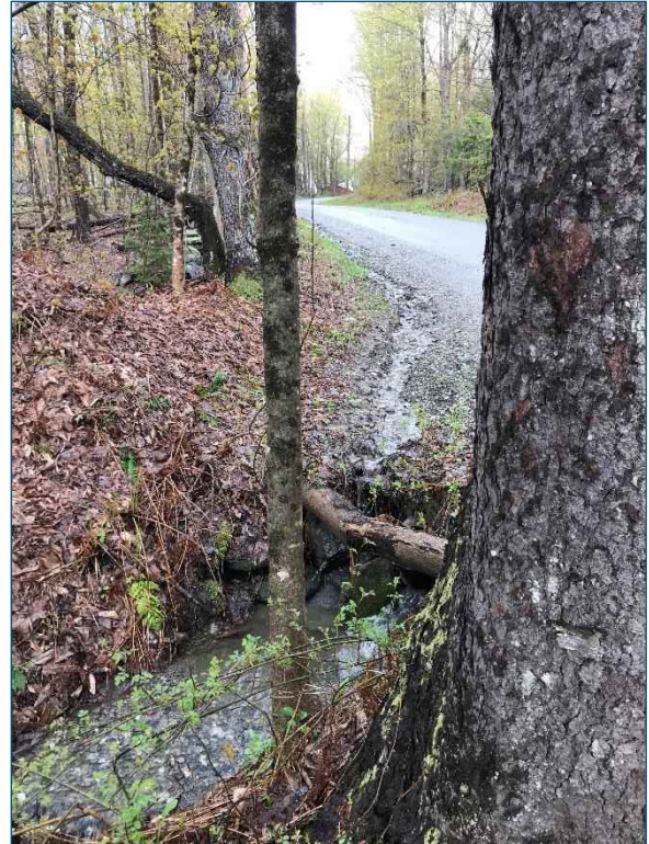
False ditch discharging directly to a stream at a stream crossing.
