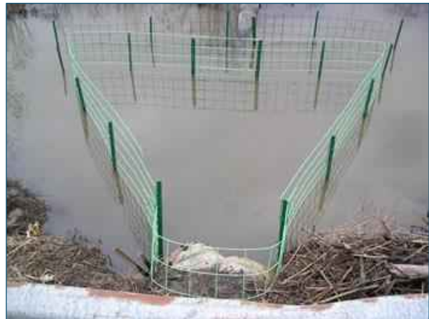
Culvert protective fence. Photo credit: Beaver Solutions.
