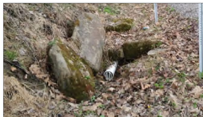
Underdrain outlet with crush resistant drain pipe, animal guard to prevent clogging, and large rocks and posts to keep vehicles from damaging the pipe.
