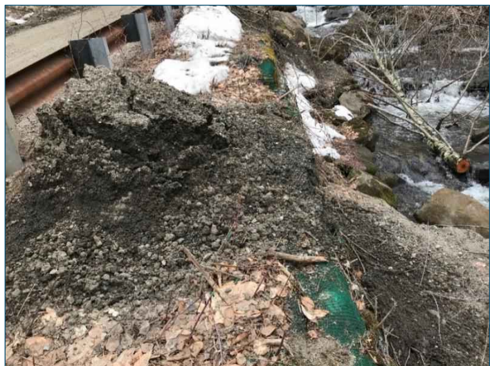
Road material from a plow pile collapsing into an adjacent brook.
