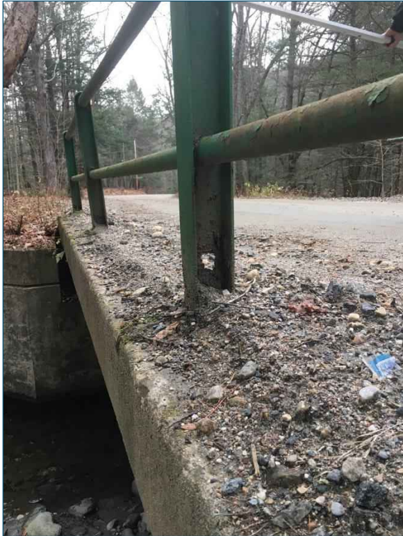
Road material loss on a bridge without berms.
