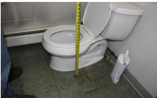
One of the two toilets in Town Hall is too short for standards.
