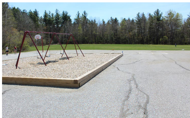
There is no cut in the border to provide an accessible pathway into the swing set area.
