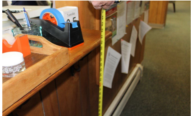
The service counter is not in compliance with standards.
