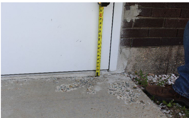
Wear and tear on the concrete created a change in level at the entrance to the building that exceeds 1/4".
